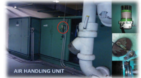
AIR HANDLING UNITS
